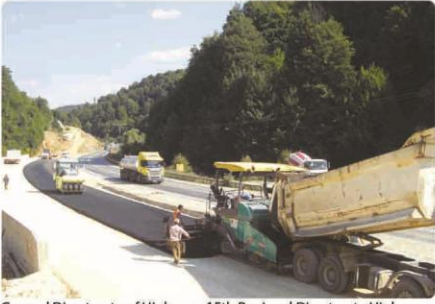
General Directorate of Highways 15th Regional Directorate Highways, Zonguldak, Bartın, Karabük, Kastamonu / Turkey
